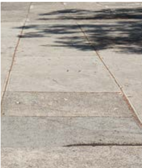
Existing concrete to be repaired
