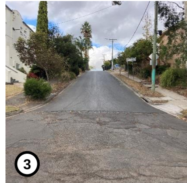
Inconsistency of surface: McArthur Rd (sealed) with The Boulevard (unsealed)
