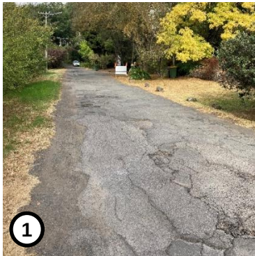
Poor condition of The Boulevard road surface
