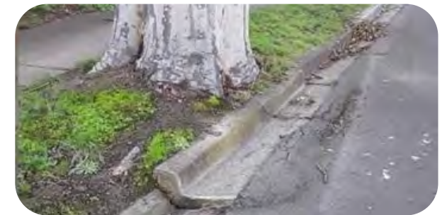
Figure 11. Poor soil depth, small planting footprint and compacted soils cause damage to footpaths. Source: Banyule City Council
